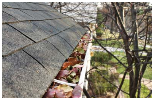
To effectively remove water from the roof, gutters need to be kept clear of debris. This photo shows clogged gutters; water will overflow when gutters are not kept clear of debris.
