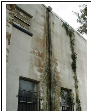
This photo illustrates a missing downspout. The water damage to the building includes algae growth and cracks in the block walls. Regular inspections looking for missing downspouts would have prevented this condition.
