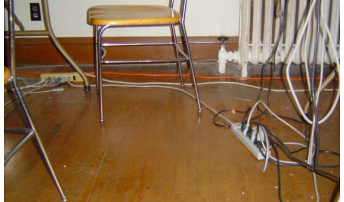
This image shows two power strips that have been plugged into each other, also called daisy chaining. This practice should not be permitted.
