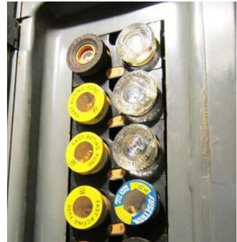
Typical screw-in fuse panel.
